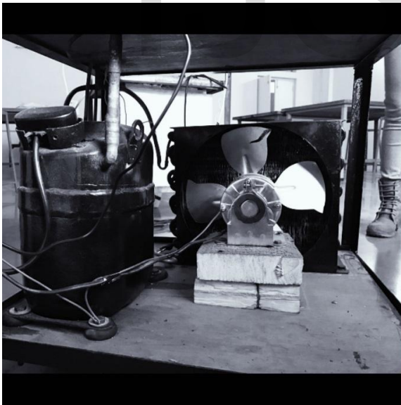
Fig. 1- Compressor and condenser
